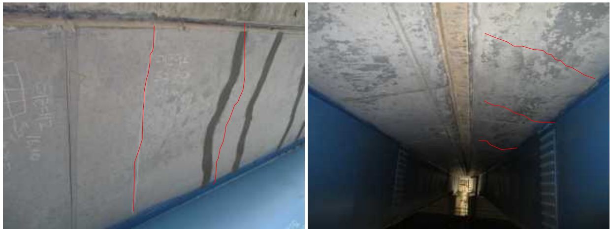
S3캔틸레버 균열(0.3mm미만)(CW=0.2/L=0.7) S2캔틸레버 균열(0.3mm미만)(CW=0.2/L=0.7)
